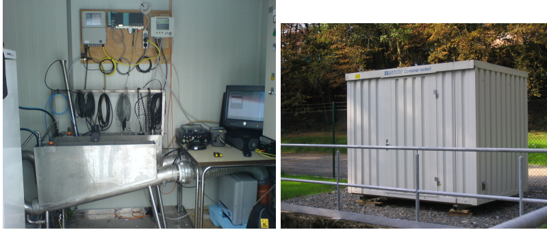
Fig. 1.14 Rain gauging station which collected the 150,000 data points.
